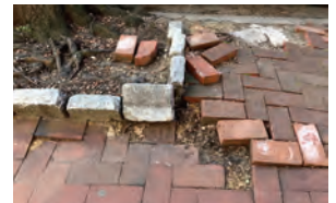
Loose bricks like these can cause trips, so get them fixed!
